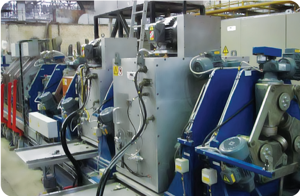
An installation at a large European tube mill featuring both longitudinal and transverse Rotoflux® rotaries to test to a 5% or 10% notch level on common OCTG products in a size range of 50 - 180mm (1.97" - 7") diameter. Inspection complies with API 5CT - Rev 8 specifications. The Longitudinal flux leakage unit includes rotating magnet poles and sensors. The Transverse unit places the magnet poles in a fixed position perpendicular to the axis of the tube.
